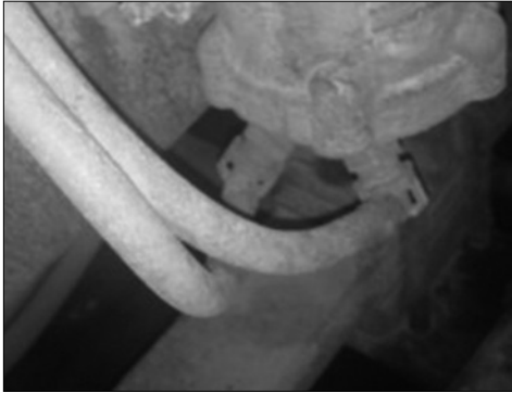
Figure 10: Voss Fitting on Bottom of Fuel Pro
